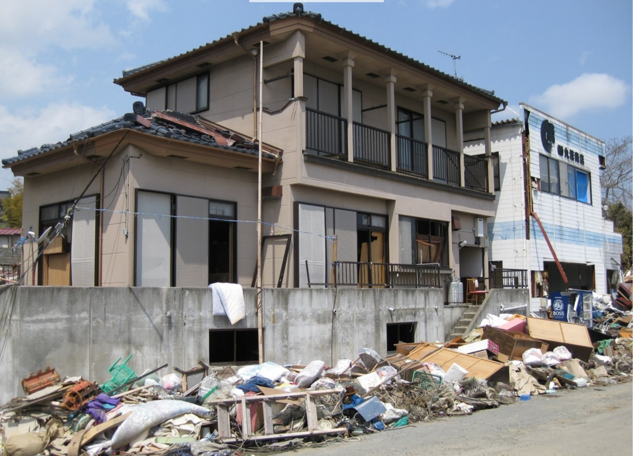
A house beyond repair
